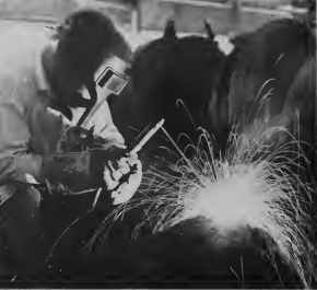
HOT SPARKS , intense glare are no friends of Lago's welders. Working safely to these employees means wearing a face shield with special glass and welder's gloves. A hard hat completes the protective gear.
